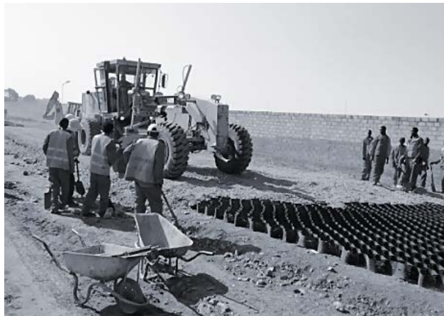
Urban Roads Upgrade, Lot 9, Matero. Layerworks, Ancillary Works and Surfacing of Urban Roads in Matero Township, Lusaka
